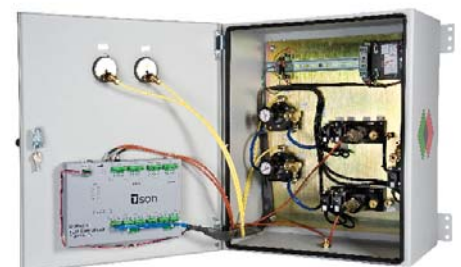
TCU2 is installed in pneumatics cabinet
